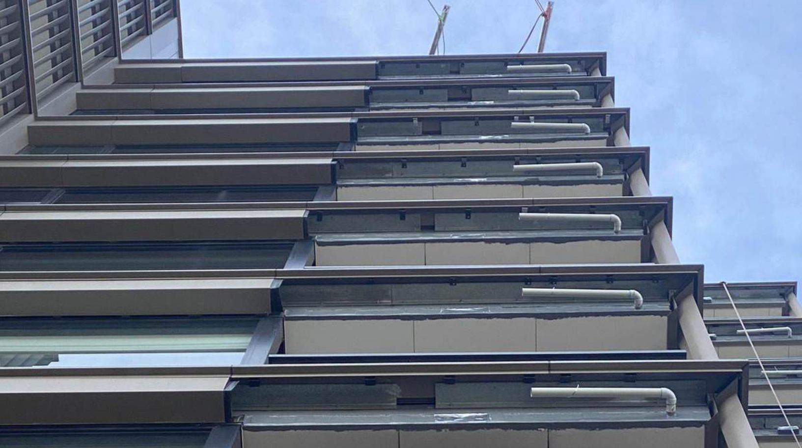
Integrated panels with each apartment's exhaust system.
